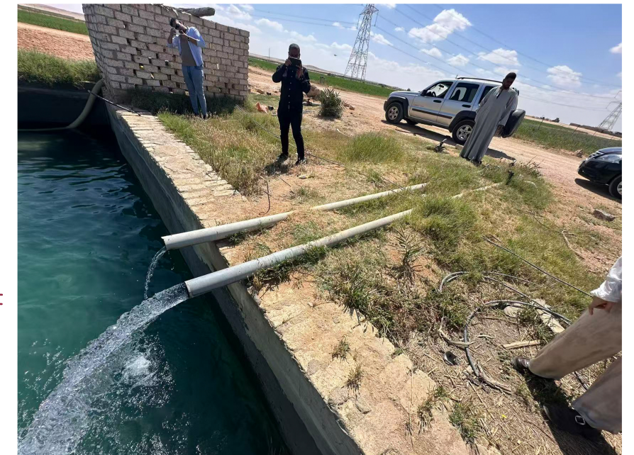
Solar Water Pump
