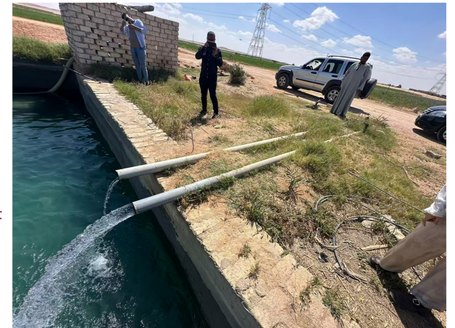
Solar Water Pump
